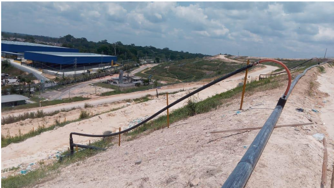
Figure 3 – Example of transmission pipelines.
